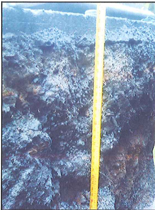
Photo 1 – Many roads within the Village were constructed on organic fill. This photo shows a section of road underlain by 1200 mm of organic material.
